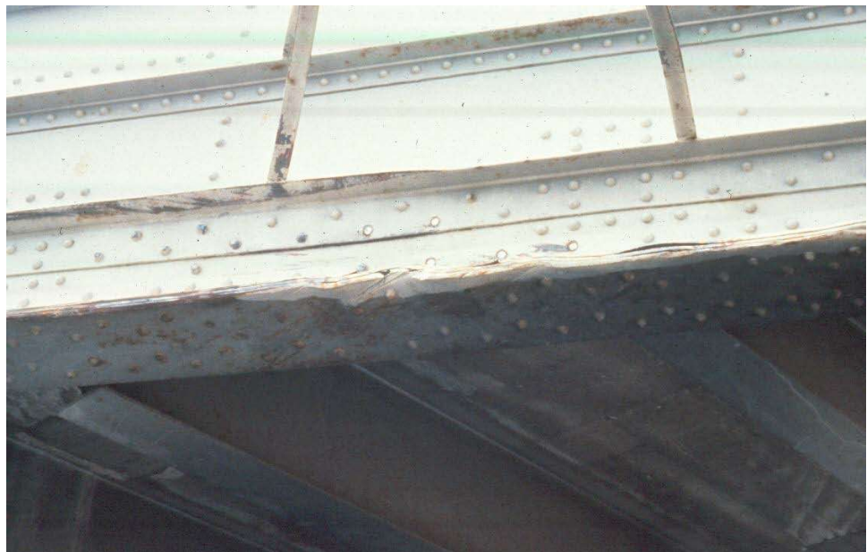
Figure 10.2.19 Collision Damage to a Through Girder Bridge
