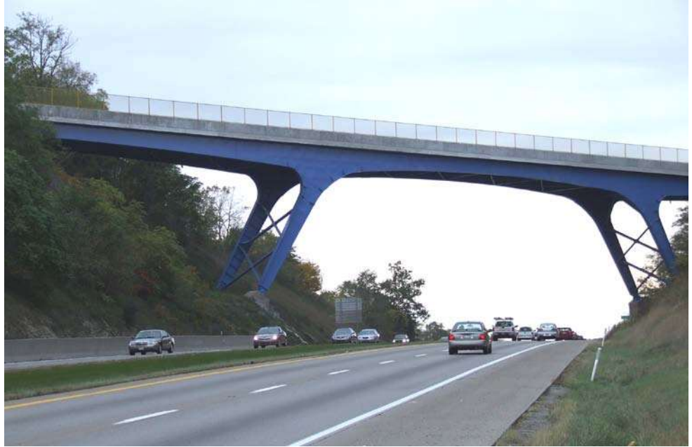
Figure 10.6.11 Fracture Critical Structure - No Load Path Redundancy
