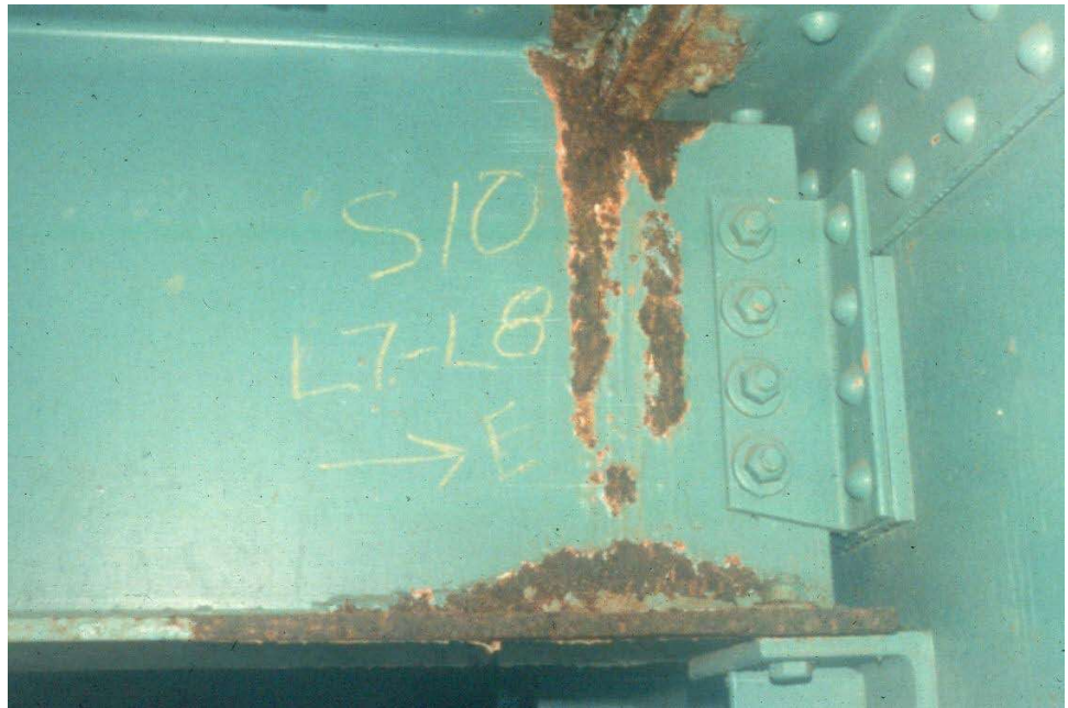
Figure 10.4.54 Corroded End of Stringer
