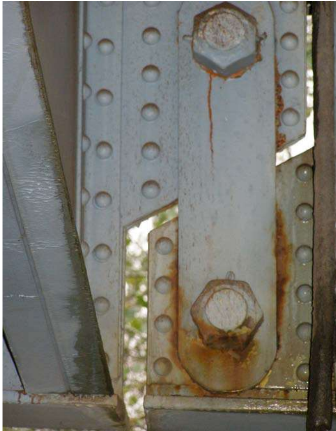
Figure 10.7.20 Rust Stains from Pin Corrosion
