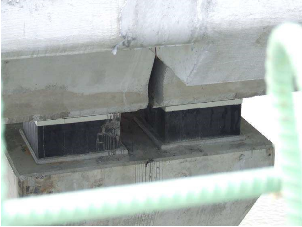
Figure 9.11.44 Segmental Box Girder Bearings at Intermediate Pier
