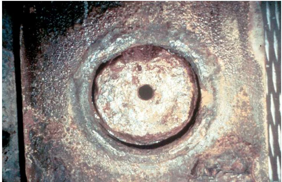
Figure 10.7.24 Corroded Pin-and-Hanger Assembly
