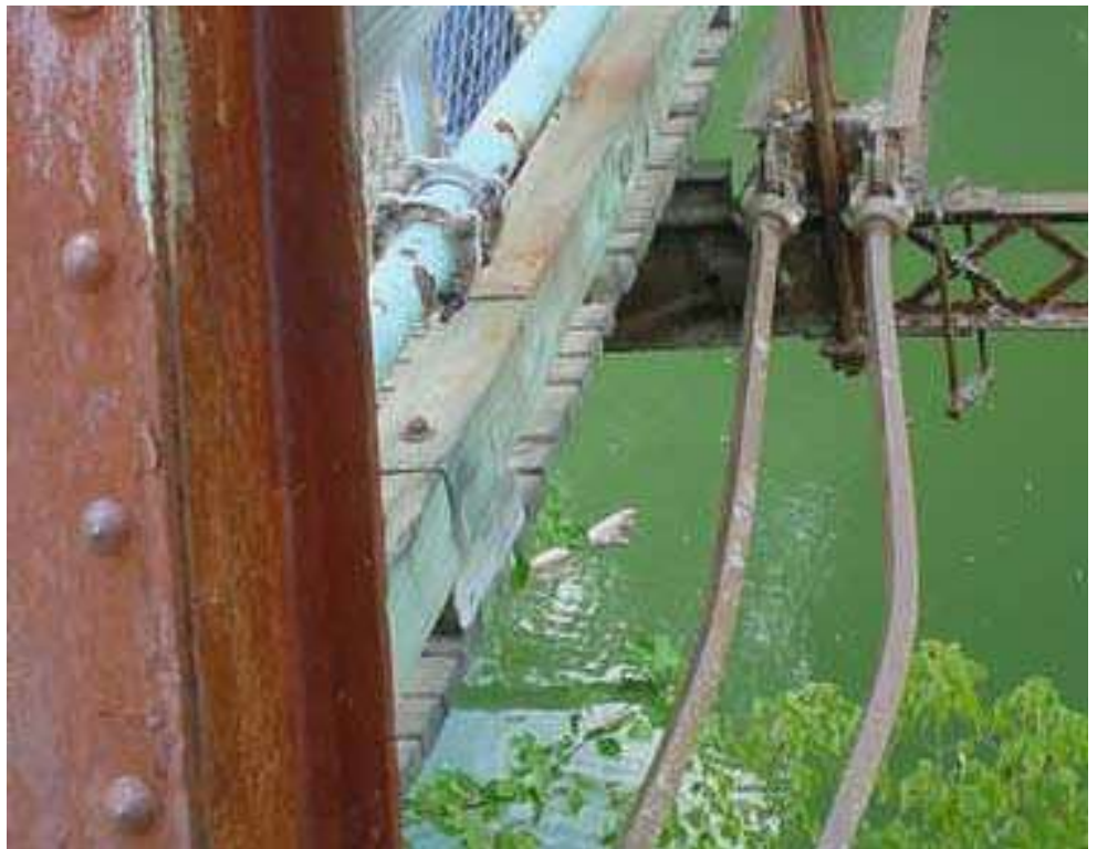
Figure 10.4.47 Bowed Bottom Chord Eyebar Member
