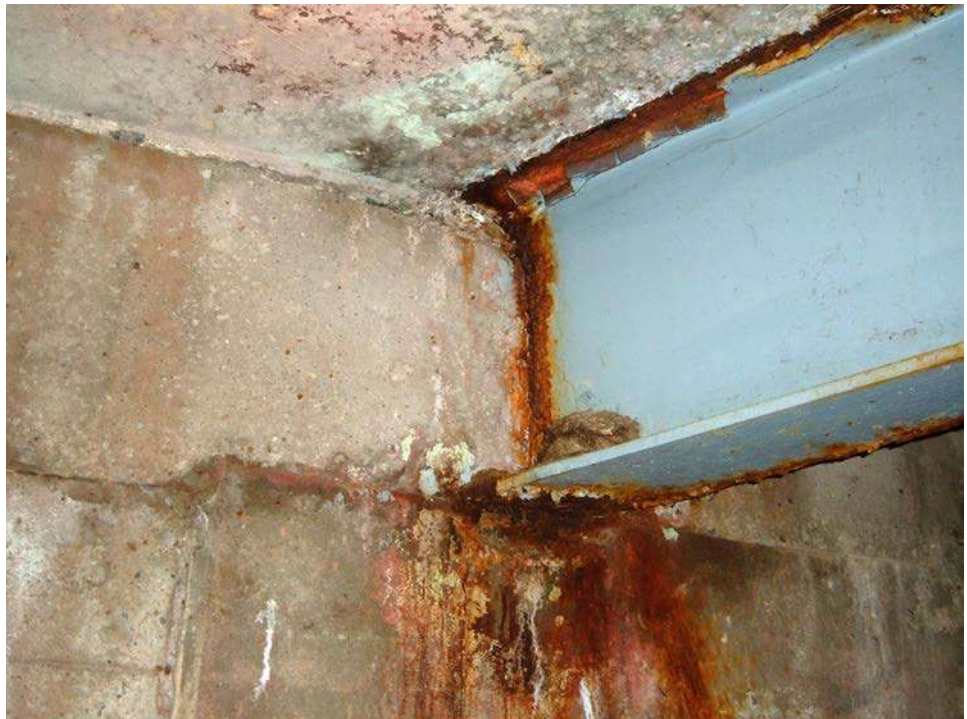
Figure 10.1.16 Corroded Shear Zone on a Rolled Multi-beam Bridge
