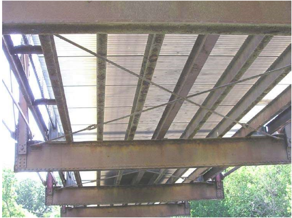
Figure 10.4.53 Corroded Stringers under an Open Grid Deck
