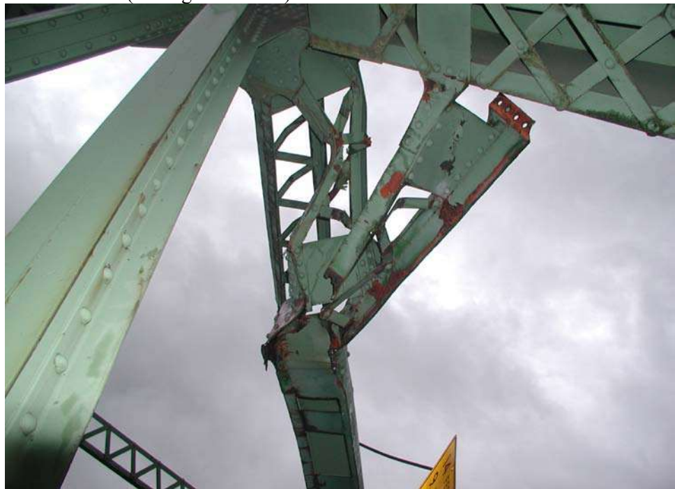
Figure 10.4.56 Collision Damage to Portal
