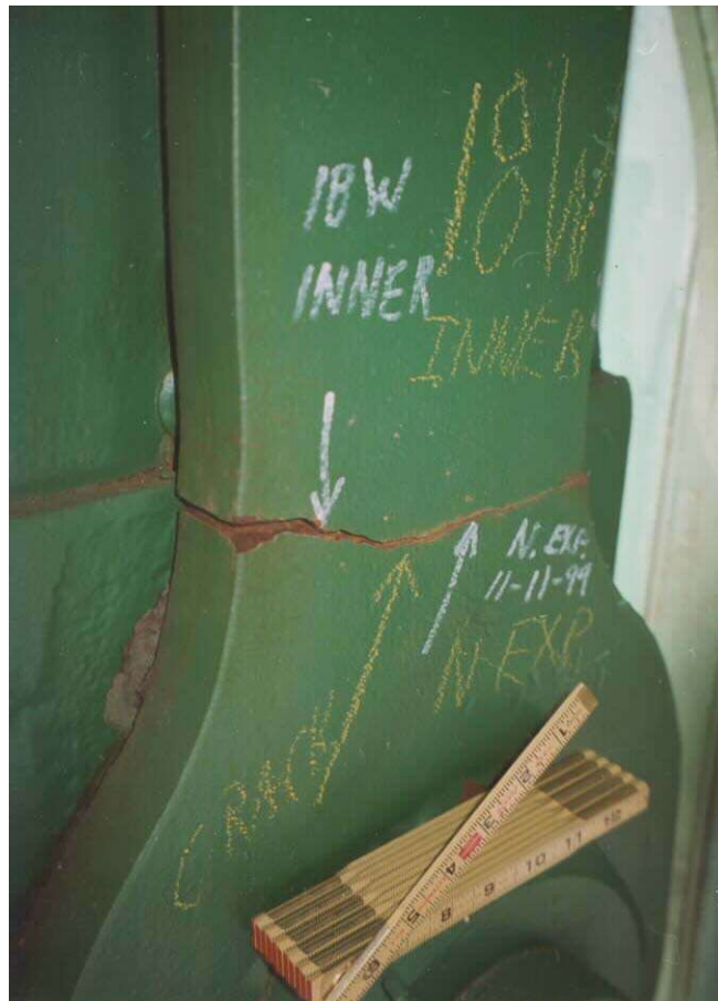
Figure 10.4.43 Cracked Forge Zone on an Eyebar
