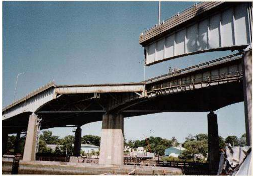
Figure 10.7.15 Mianus River Bridge Failure
