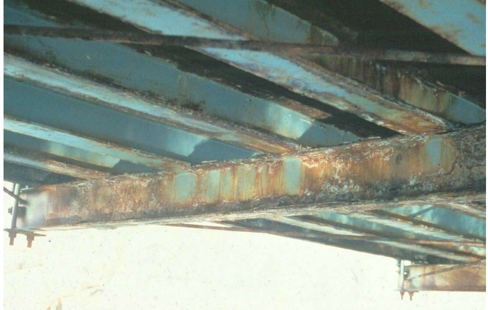
Figure 10.4.55 Corroded Floorbeams and Stringers
