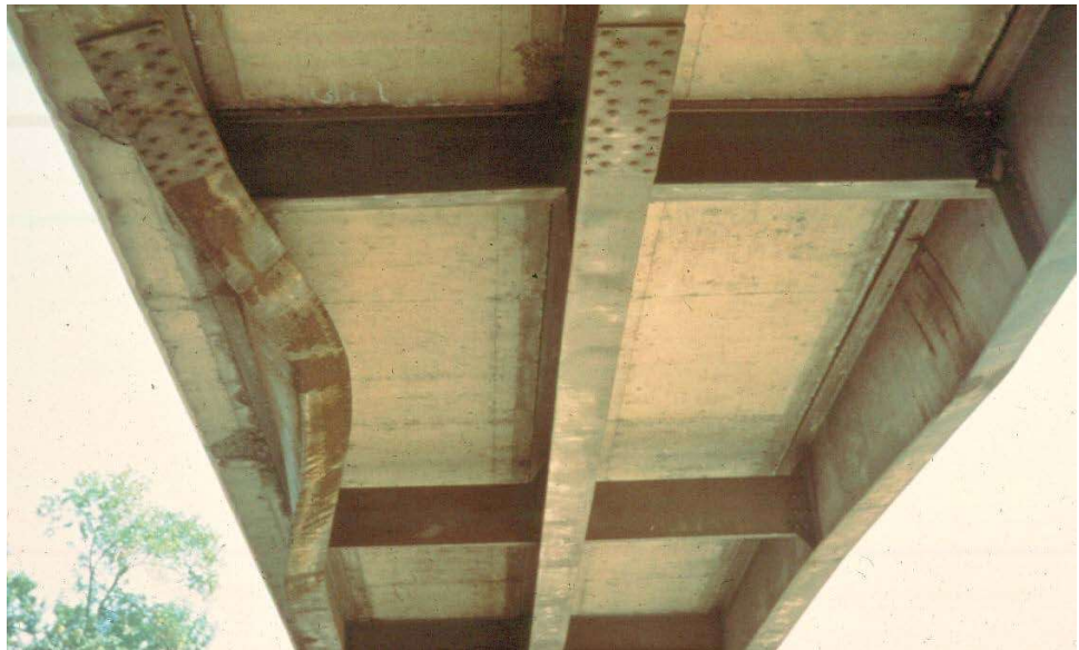
Figure 10.1.24 Collision Damage on a Fabricated Multi-Girder Bridge
