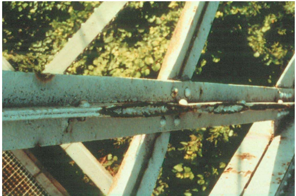
Figure 10.4.58 Sway Bracing with Pack Rust
