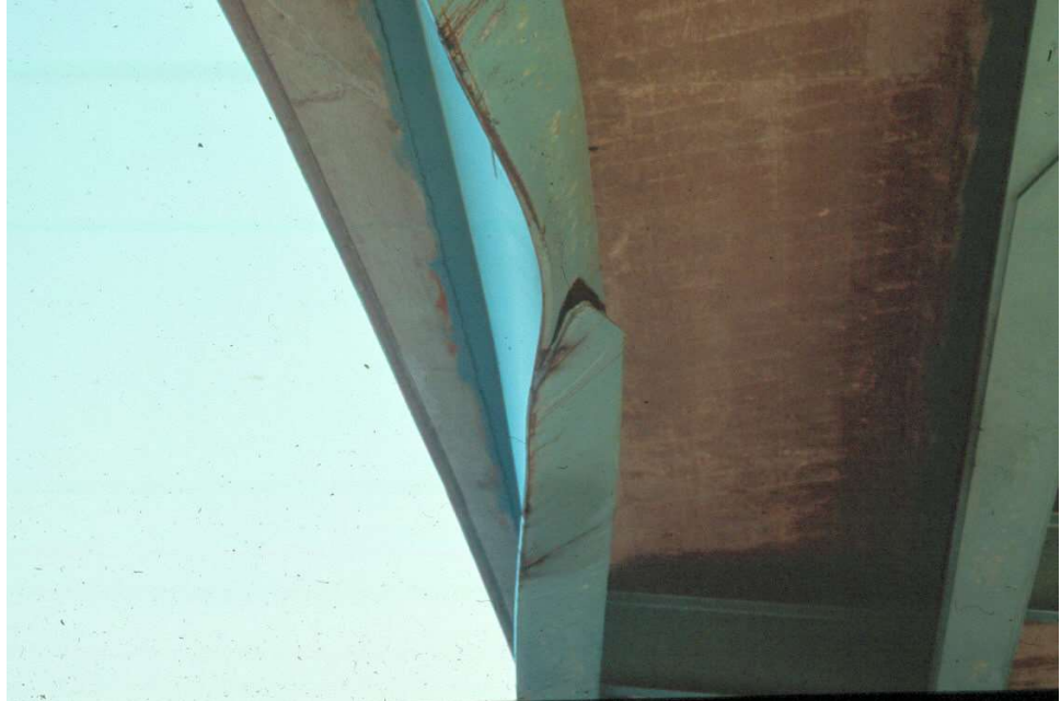
Figure 10.1.23 Collision Damage on a Rolled Multi-Beam Bridge
