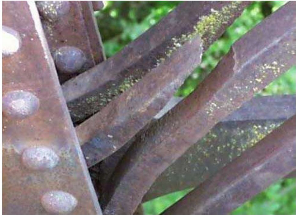
Figure 10.4.44 Cracked Forge Zone on a Loop Rod
