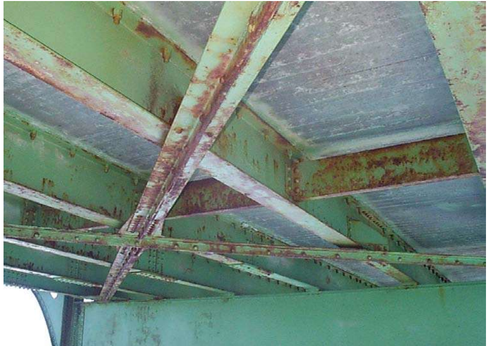
Figure 10.4.57 Lateral Bracing with Corrosion
