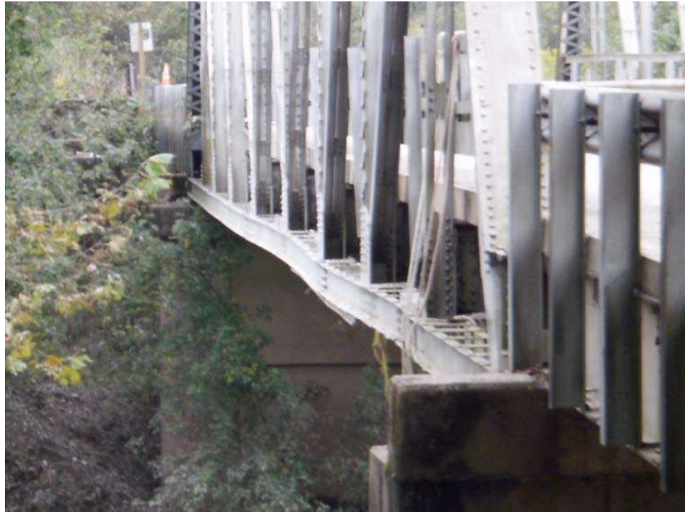
Figure 10.4.48 Buckled Bottom Chord Member, Due to Abutment Movement
