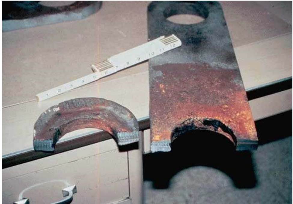
Figure 10.7.21 Corroded Hanger Plate
