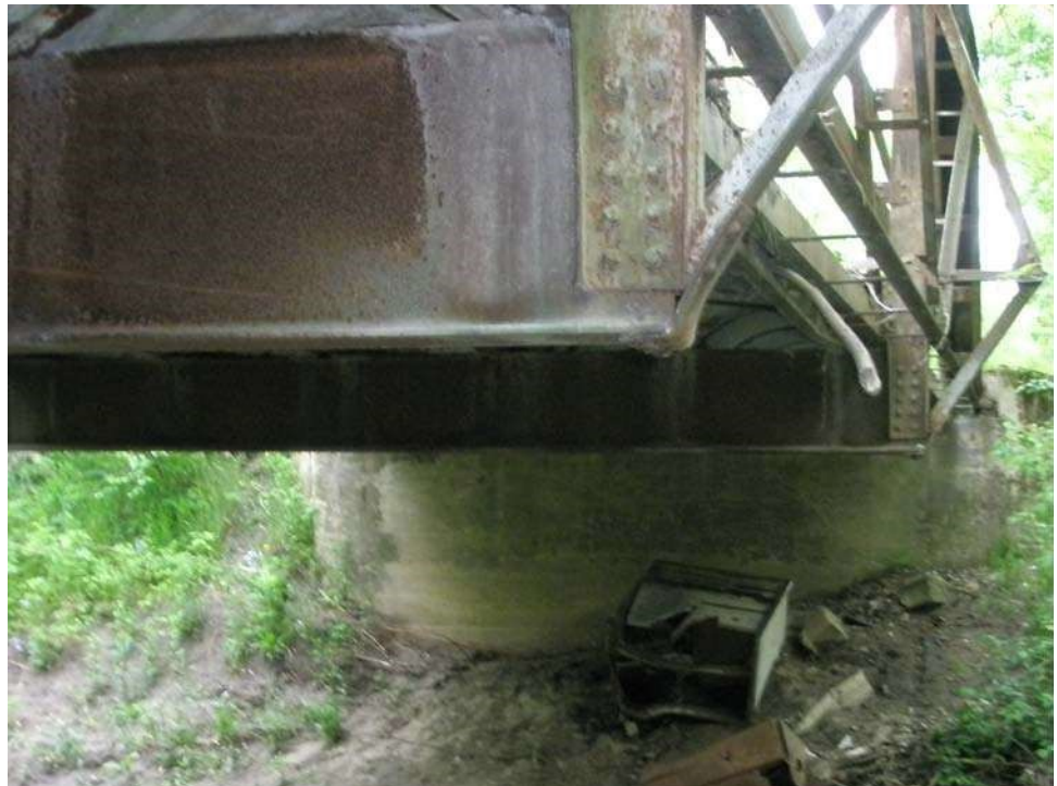
Figure 10.4.52 Corroded Floorbeam End and Connection with Deicing Chemical Residue
