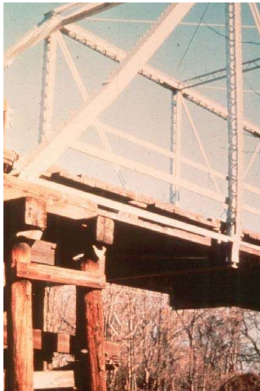
Figure 10.4.50 Buckled End Post
